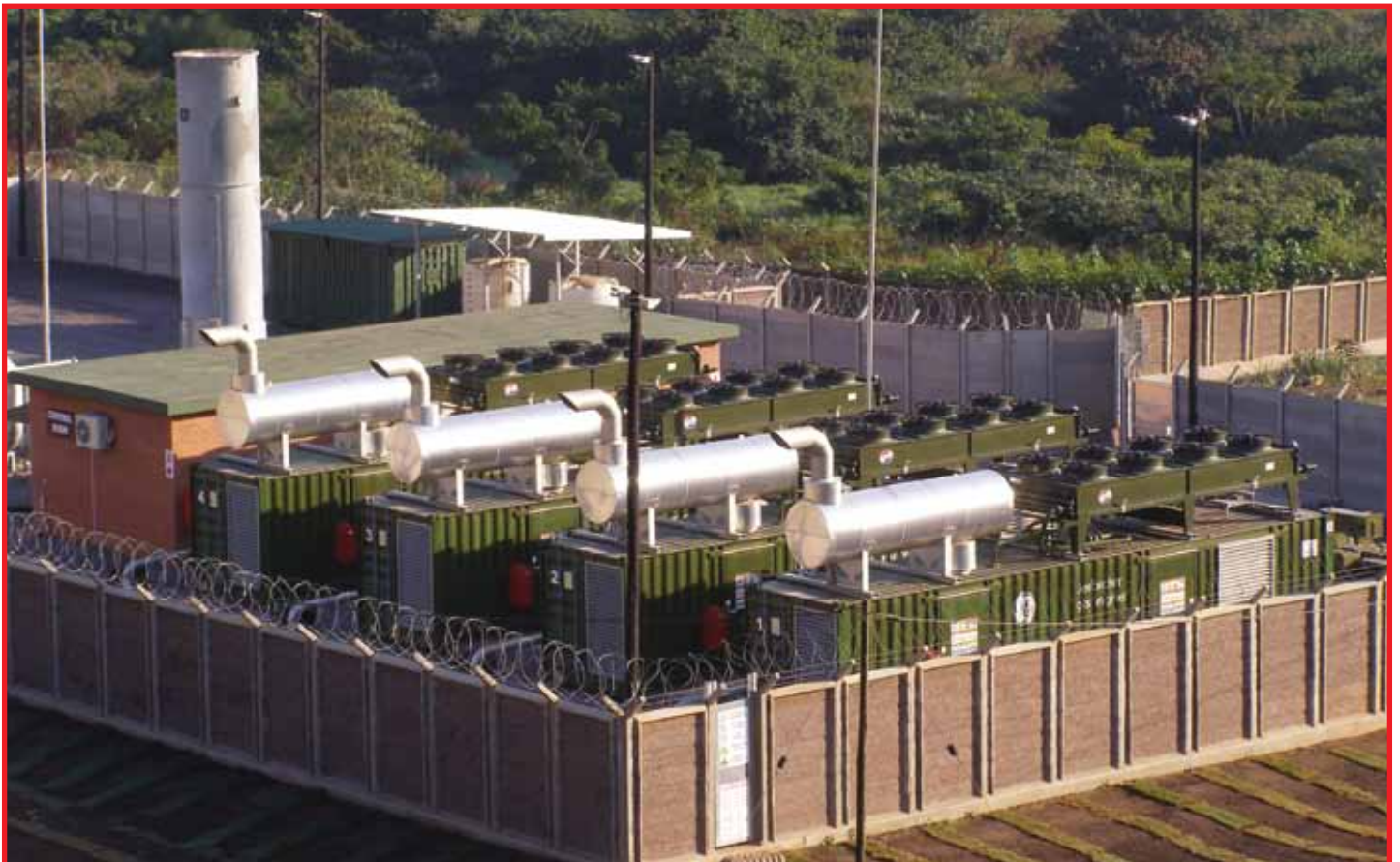
Durban solid waste landfill gas to electricity plant courtesy of Clark Energy
